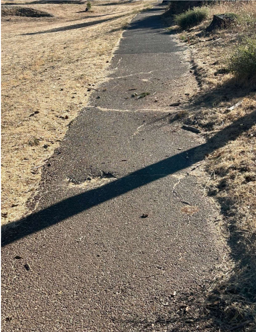
Marked for replacement
