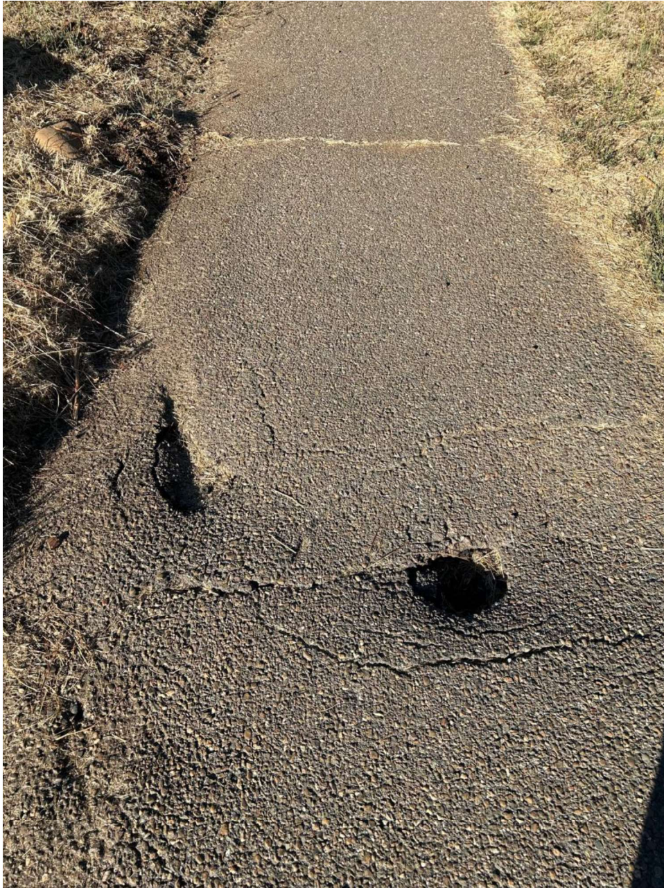
Example of walk & bike path damage – section to be torn out & restored
